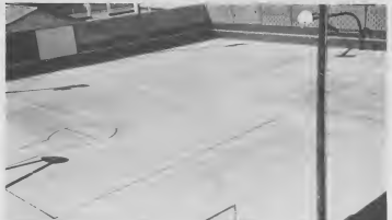
THE ENTIRE court area of the Lago Sport Park facilities was renewed with a five and one-half-inch layer of concrete. The huge pour was completed at the end of the year, which allowed time to organize the island-wide volleyball tournament as the first activity on the new surface. Ten girls' teams are participating in the play.
